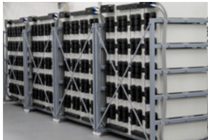
Energy Storage System
